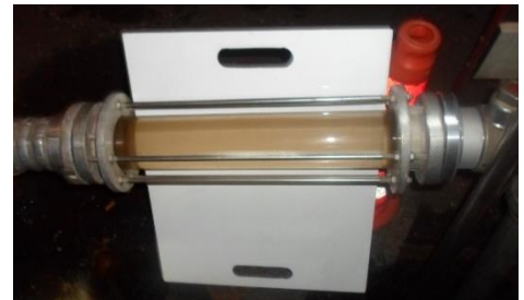
Figure 3: turbidity in inspection glass during cleaning process
