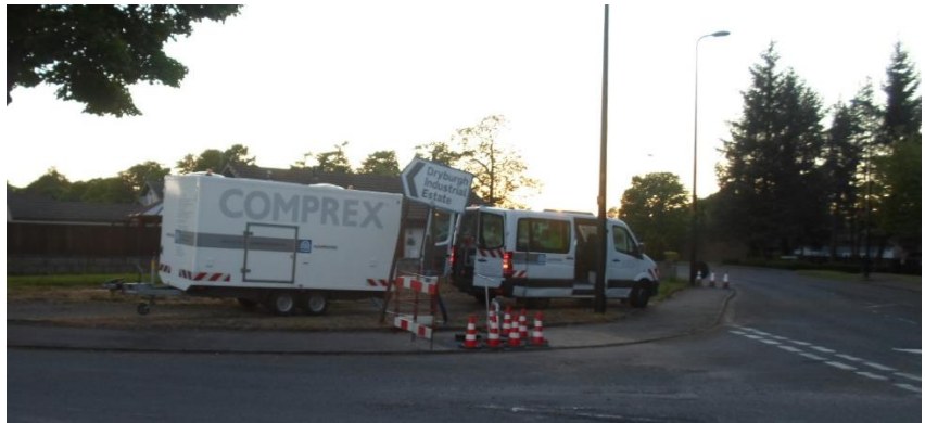
Figure 1: Comprex® equipment on site
