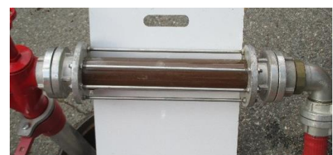
Figure 4: turbidity in inspection glass during cleaning
