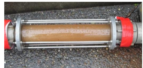
Figure 4: inspection glass for visual monitoring of the progress of cleaning
