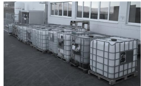
Figure 3: discharge via IBC
