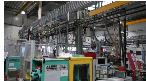
Figure 2: pipeline system at the injection molding machines
