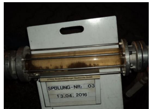
Figure 4: Inspection glass at discharge location
