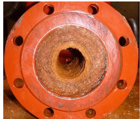
Figure 2: Condition of pipe before cleaning
