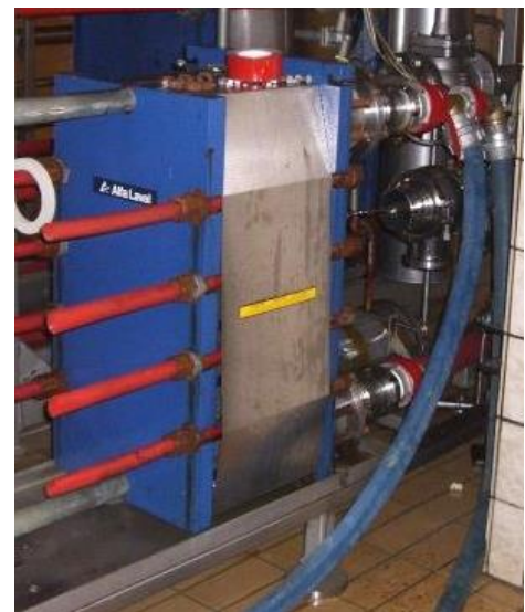
Figure 2: gasketed plate heat exchanger
