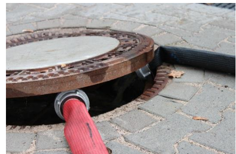
Figure 4: discharge into drain shaft
