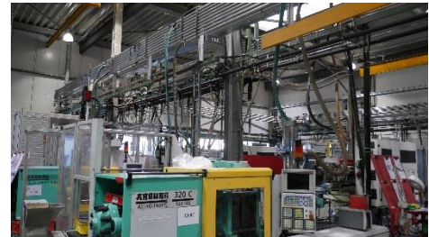
Figure 2: pipeline system at the injection molding machines
