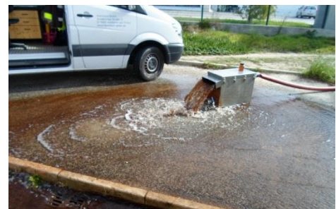
Figure 3: turbidity at discharge box
