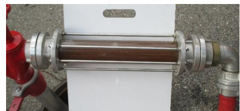
Figure 4: turbidity in inspection glass during cleaning
