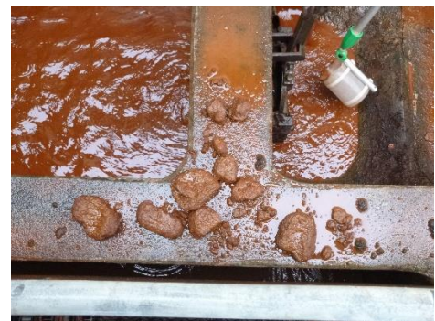
Figure 4: Water outlet at settling tank
