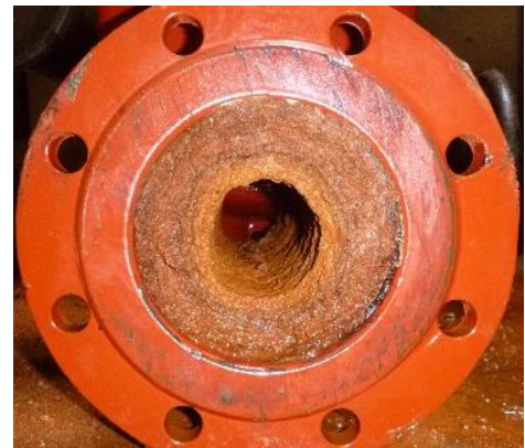
Figure 2: Condition of pipe before cleaning
