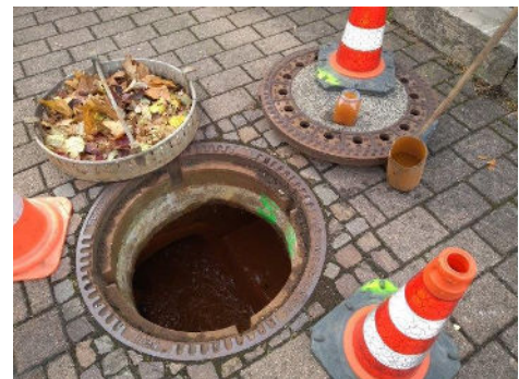
Figure 3: Monitoring water discharge
