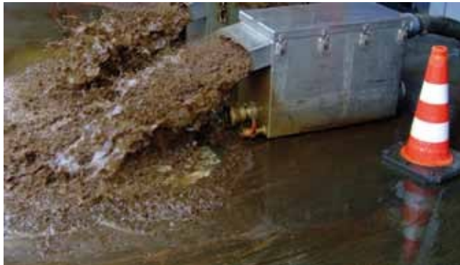
Fig. 10: Rinsing water discharge via rinsing boxes during Complex cleaning of DN 250 supply and return pipes
