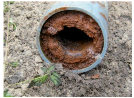
Figure 5: Iron sludge in plastic pipe Fig. 5: Iron sludge in a plastic pipeline
