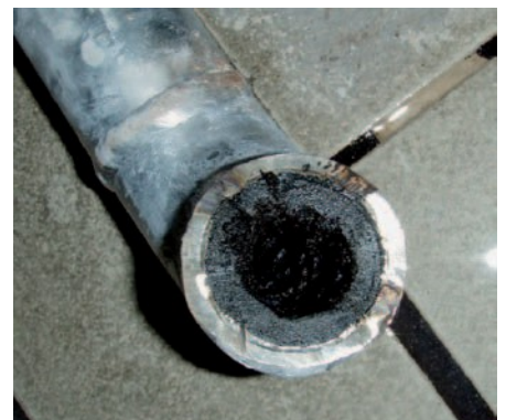
Figure 6: Manganese sludge in stainless steel piping Fig. 6: Manganese sludge in a stainless steel pipeline
