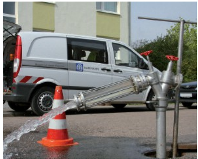
Fig. 2: Non-closing gate valve, recognizable by the water leakage
