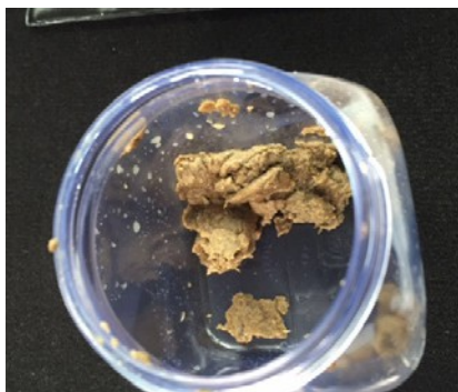
Figure 4: Deposits discharged from the cooling system (example 1)
