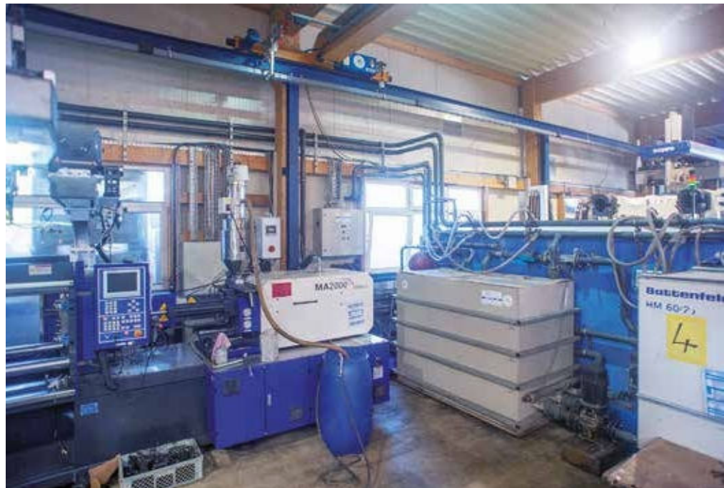
At Wefoba, a ring main supplies machines and tools with cooling water. Connections for water purification and the physical water treatment system are located in the central supply line. A free cooler relieves the load in winter.
