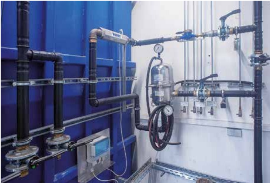
The system for physical water treatment (installed horizontally at the top) is integrated into the self-sufficient cooling circuit of the extrusion system.
