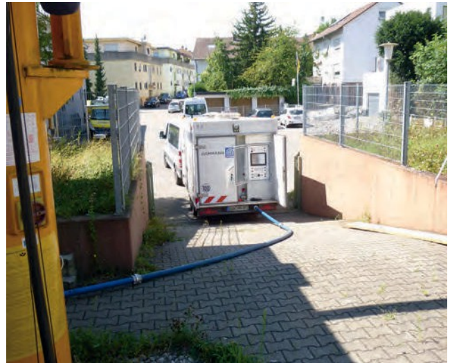
Fig. 1: The technical cleaning unit at the pumping station
