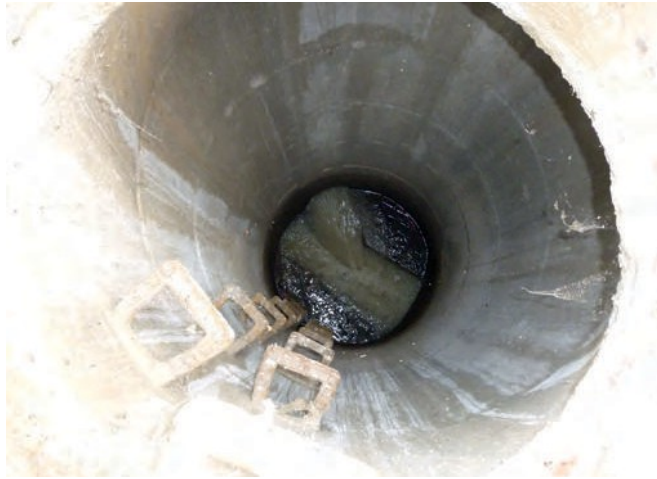
Fig. 4: Discharge into a gravity sewer
