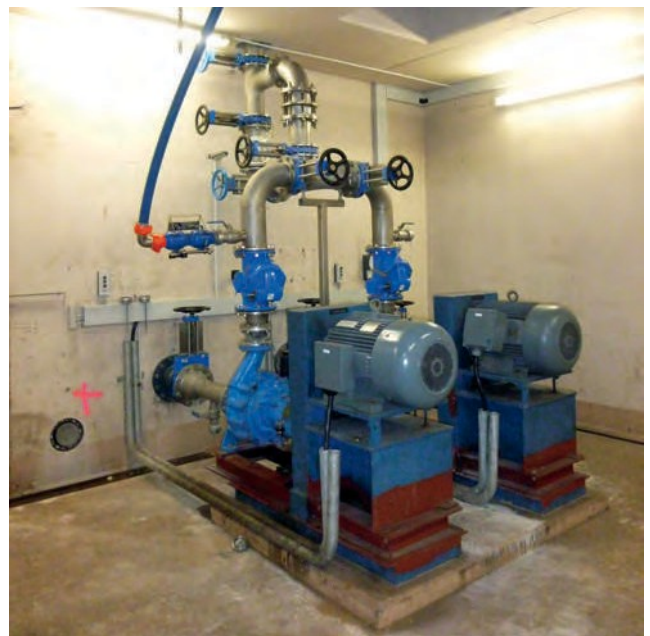
Fig. 2: Feed point via pump
