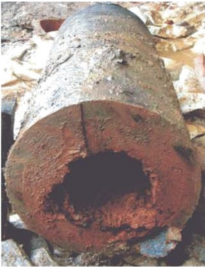
Fig. 9: Deposits in the AZ connection pipe of well 1
