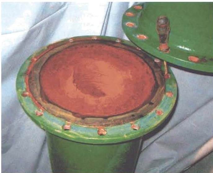
Fig. 10: Deposits in a steel pipe in the waterworks Weather field
