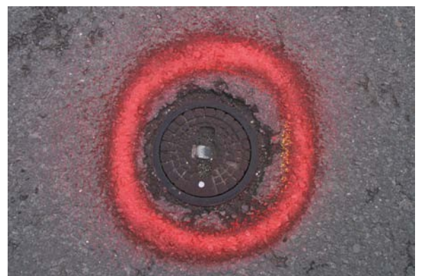
Fig. 6: Marking on the steel cap after upgrading: green (upgraded), red (defective)
