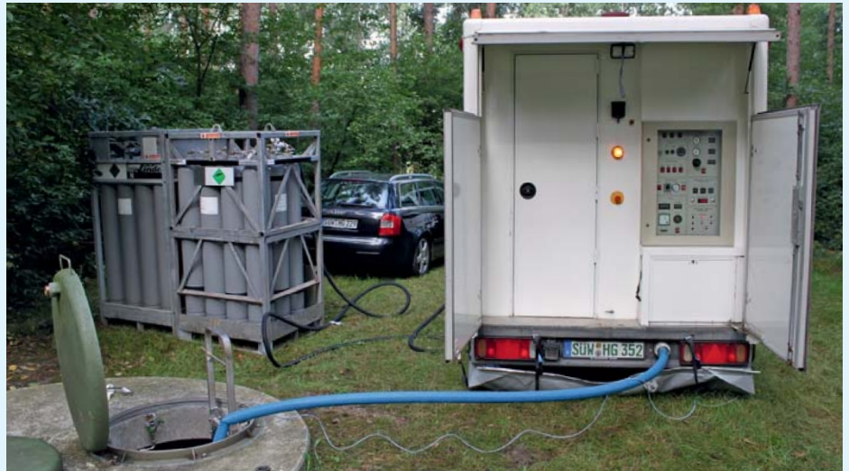
Figure 5 Compressed air and nitrogen feed into the well line controlled by a Complex unit
