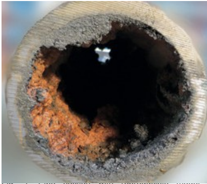
Fig. 1: Pipe section with reproducible model deposits (top) and pipe section from practice with deposits (bottom)
