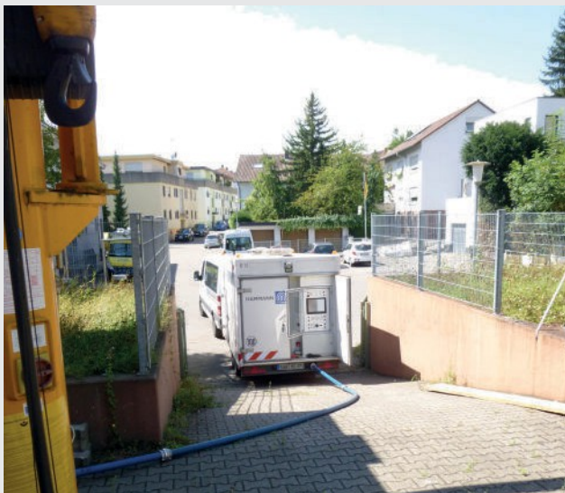
Figure 4: Complex unit at pumping station
