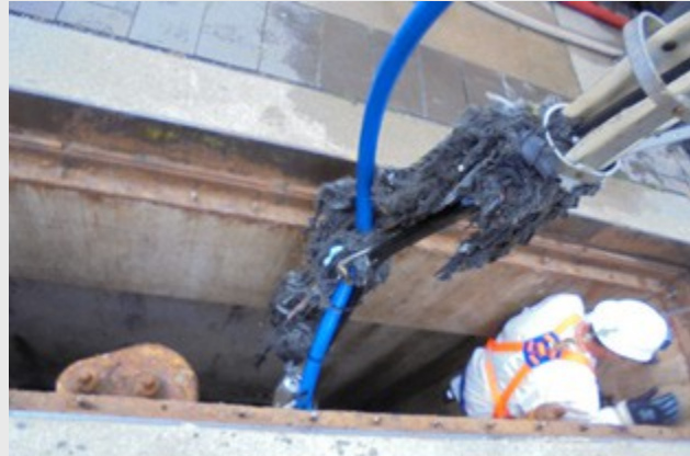
Figure 7: Pulling out the black rinsing hose with rinsing nozzle and attached blue PE pipe as well as accumulation of adhering damp cloths and nonwovens
