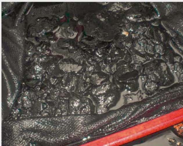
Fig. 7 Aged grease deposits from waste water pressure pipe after cleaning
