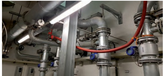
Fig. 5: Compressed air feed in the Küssnacht pumping station
