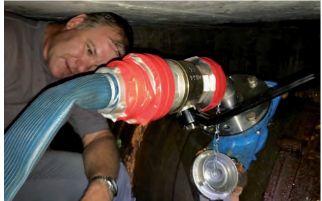
Fig. 4: Compressed air connection at the intermediate feed point
