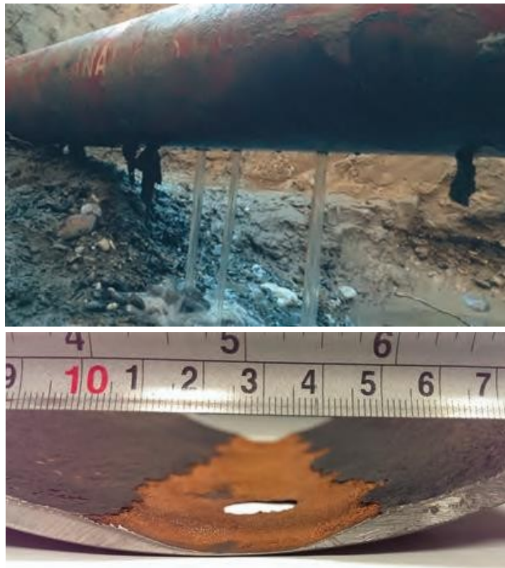
Pipe breakthroughs due to abrasion caused by coarse particles in the sole area
