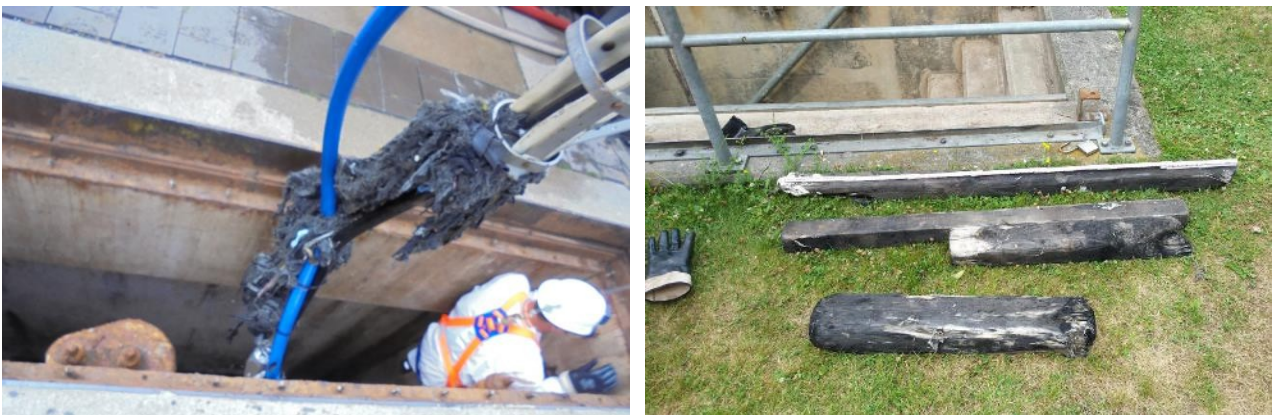
Wet wipes, nonwovens and wooden parts from culverts
