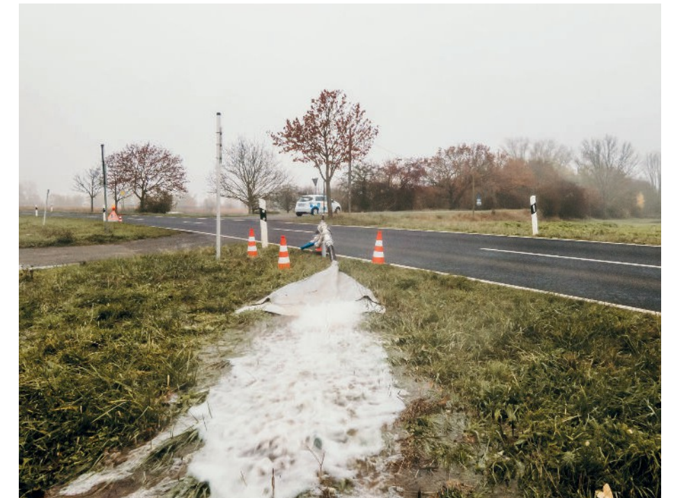
Figure 7 Discharge at the outlet point Source: Hammann GmbH
