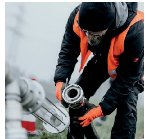
Fig. 6 Sight glass at the outlet point for inspection and documentation of the turbidity. Source: Hammann GmbH
