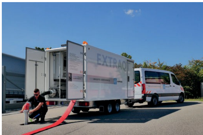
Figure 1: Units for the condition assessment and cleaning of pipes
